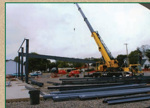
Construction of the 3rd addition which is currently the Hardware department, the cashier area and the entrance to the store. 2007-2008
